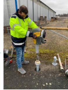
Stage 3: drive in the anchor piles using a pneumatic hammer and dedicated installation tool.
